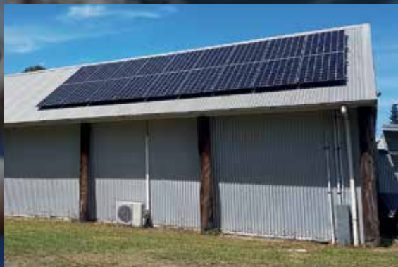
Installation of solar power at the Bundanon Artists in Residence complex. The sustainability project was supported by Clubs NSW, February 2017.
