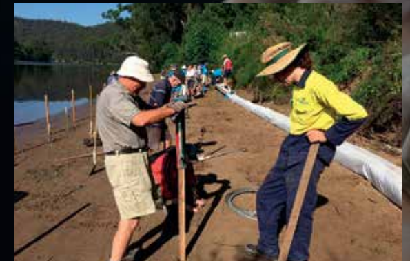
Installation of the innovative 'Sand Sausage' to prevent erosion along the Shoalhaven foreshore – in collaboration with Riverwatch, April 2017.
